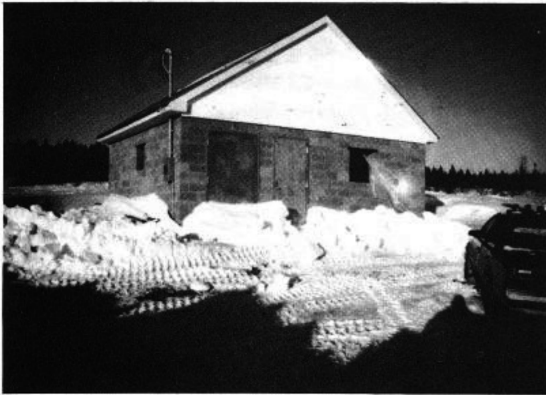
Transmitter building and 300-ft tower are being constructed on 5-acre site on Caledonia Mountain, south of Moncton.
