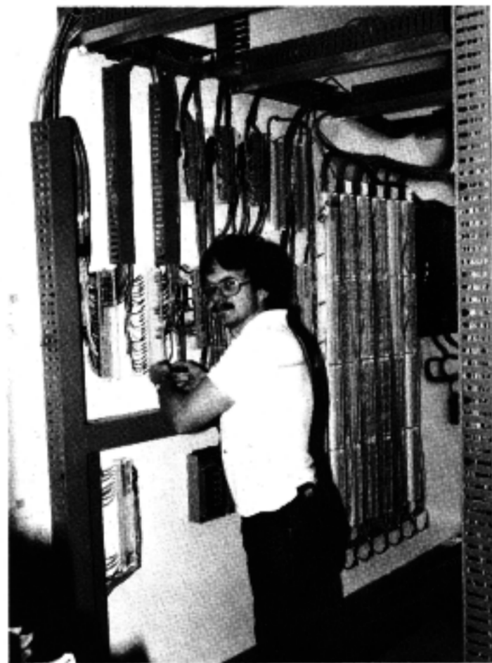
Rackroom. Chief engineer Dave Glasstetter is seen checking installation.
