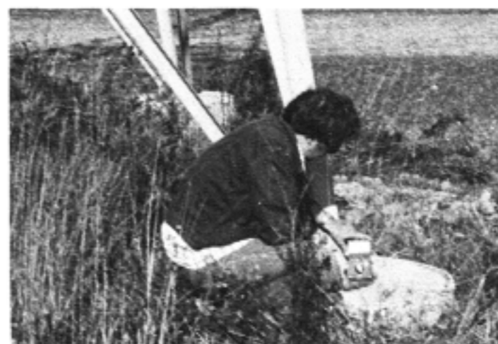
Photo 5: Bruce Dingwall holds specially-designed detuning meter against base of tower leg during detuning.
