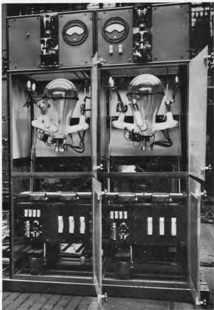
FIG. 102.—A small tramway traction equipment used to boost the pressure at the end of a track overhead line.
