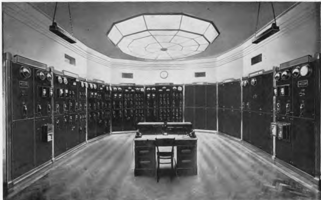
FIG. 48.—A view of a remote control switch and instrument board for a steel tank rectifier sub-station. (G. E. C.).
