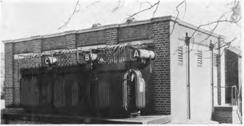
FIG. 37.—A glass bulb traction rectifier sub-station giving a 550 volt D.C. supply to a tramway system.
