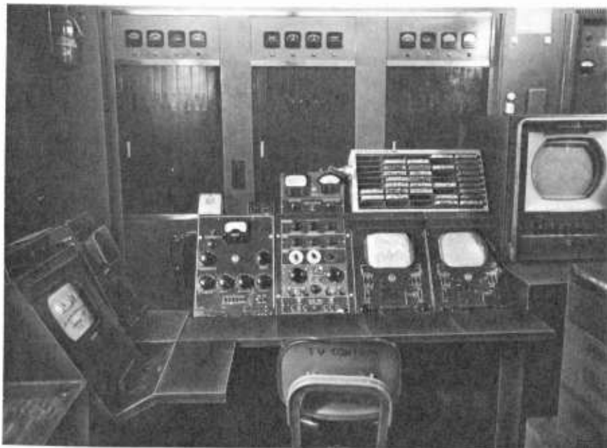
Fig. 10-5. A control room operating position designed for one-man control operation. (WLBC-TV, Muncie, Indiana)
