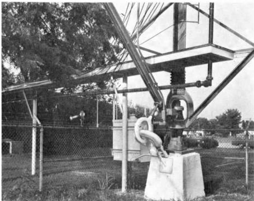
Fig. 6-17. A protection shelter for a horizontal run of transmission line. (WLBC-TV, Muncie, Indiana)
