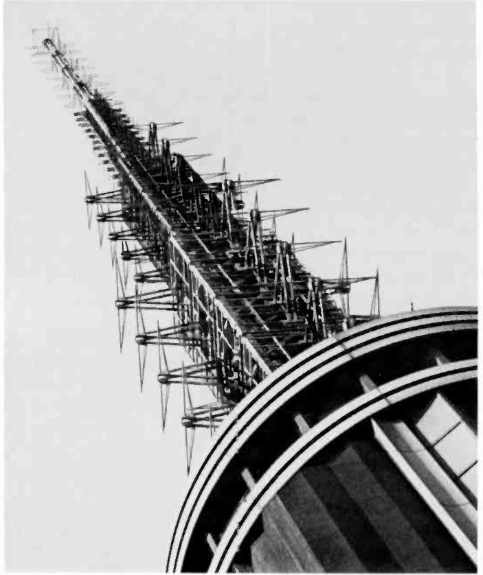
Fig. 5-9 VHF transmitter antennas atop Empire State Building in New York City.
