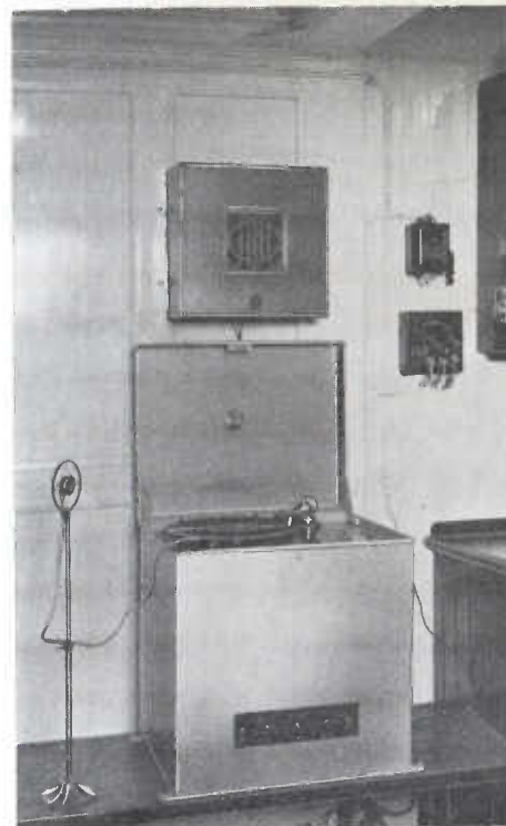
Fig. 501. Marine Band Repeater Installation Type No. 566.
