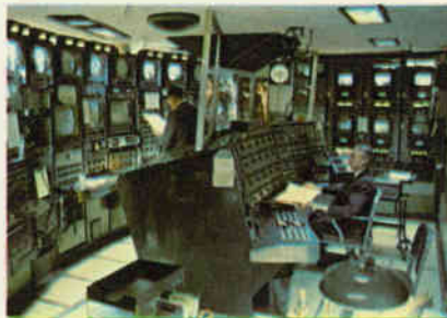
Overall master control consoles, not showing the "round robin" monitors.
