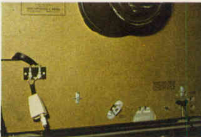
Fig. 10. Indoor transformer on TV set.
