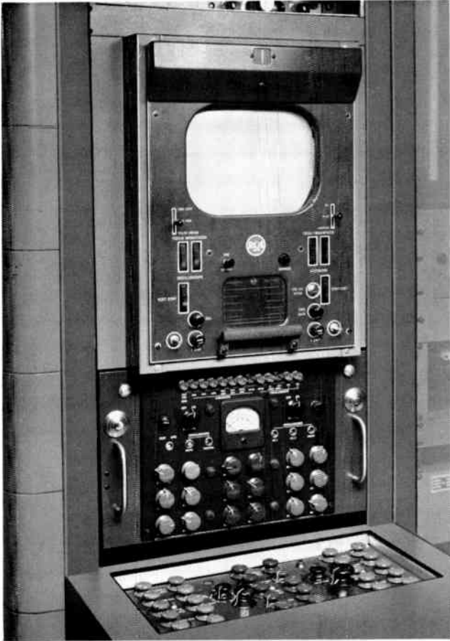
FIG. 11. Alternative method of mounting processing amplifier and master monitor in a standard cabinet rack. Camera control is shown in desk below amplifier.
