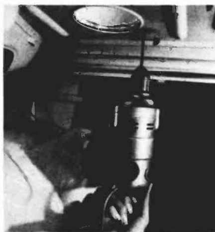
Fig. 7. Here's how it looks from inside the trunk. Note that in this car even the speaker mounting holes are pre-punched. Just drill through the rear deck cover from the trunk side. The metal tabs at the rear hold the speaker wires when they are bent upwards.
