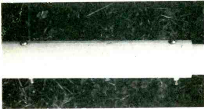
Fig #3 Bolted PVC Piping
