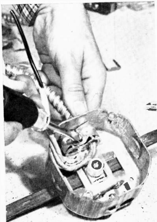
Ceiling light fixture box has a long bar that's attached to rafters. Cable is clamped by tightening the fitting screw that compresses the armor jacket.
