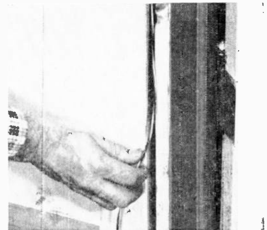
Force the 18-gauge wire between frame and wall. Keep it fairly taut so molding can be nailed flush to frame.
