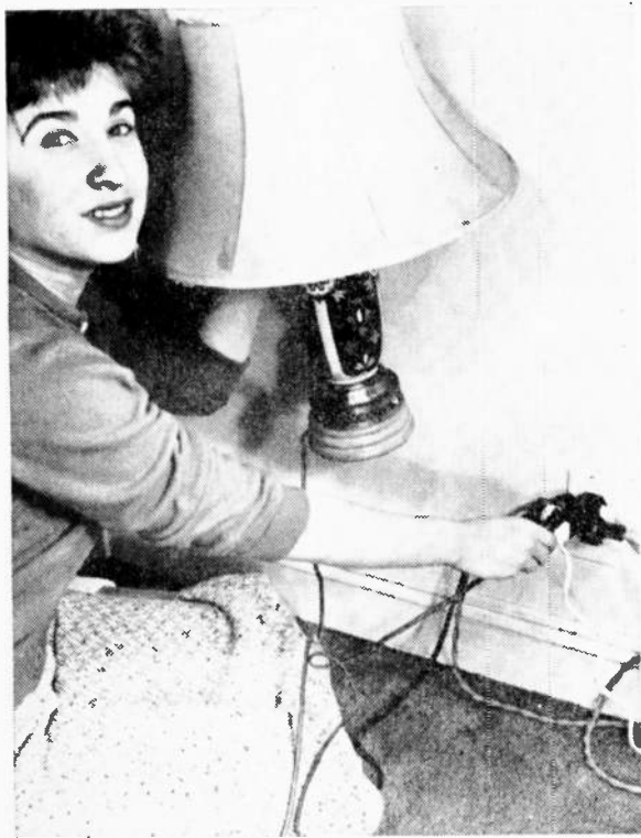
You can end extension cord clutter and install new fixtures by putting outlets where you need them. There are several methods you can use to do the job; no special tools are needed for installation.
