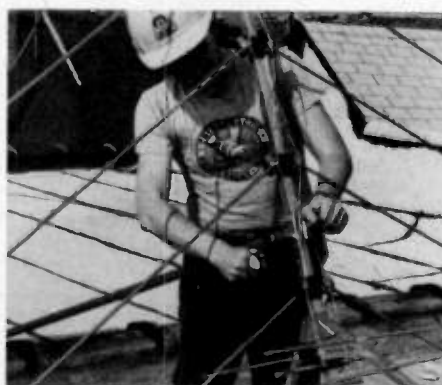
Secure the antenna to the mast. Most damage to the elements occurs at this time.
