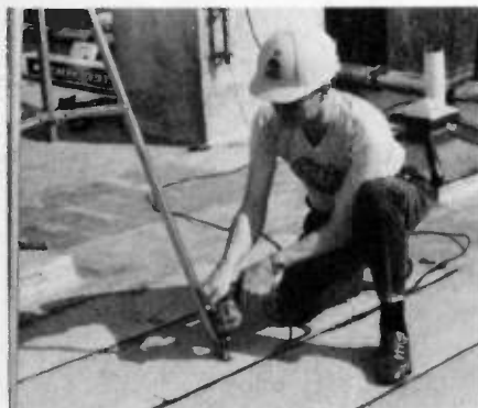
Drill pilot holes for the lag screws and make sure the tower is straight and steady.
