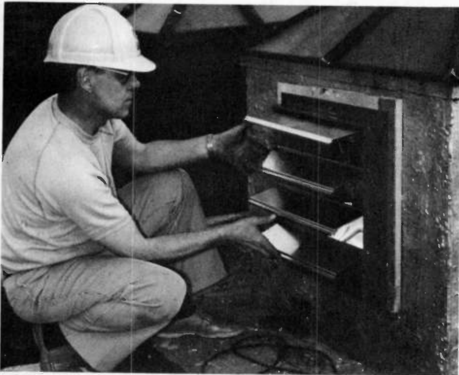
Check the operation of the self-opening louvers. Be sure that they do not bind, scrape or stick. Remove any bits of material that might cause sticking, after all you want to make certain they open everytime. Who wants to go on the roof more than they have to?
