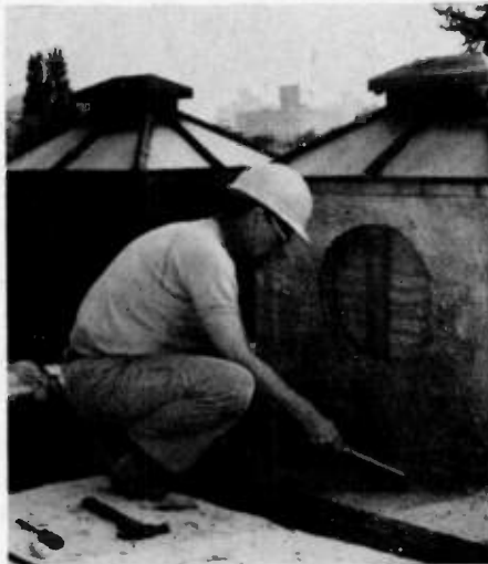
Don't let stray nails or fragments lie about on the roof. If you step on one, then there goes your roofing materials!
