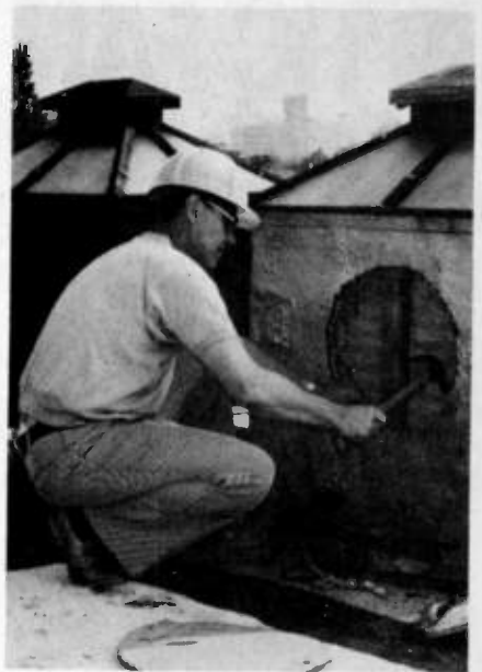
A stud and interior plaster had to be removed. We hammered away splinters and used an old drill bit to do the remainder.
