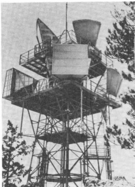
FIG. 1-26. A radio relay tower used for the reception and transmission of television signals.
