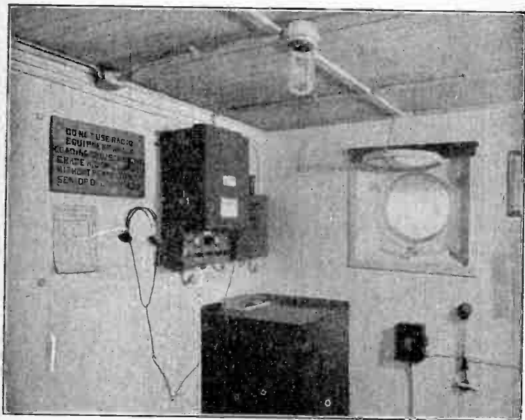
FIG. 6 —Typical shipboard installation showing location of auto alarm unit and associated equipment.
