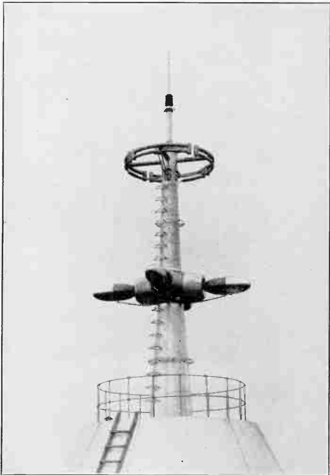
FIG. 27 —The new R.C.A.-N.B.C. television broadcast antenna as it appears on top of the Empire State Building in New York City. The antenna is located 1,200 feet or approximately one-fifth of a mile above the sidewalk of the building. The apex is a lightning rod.
