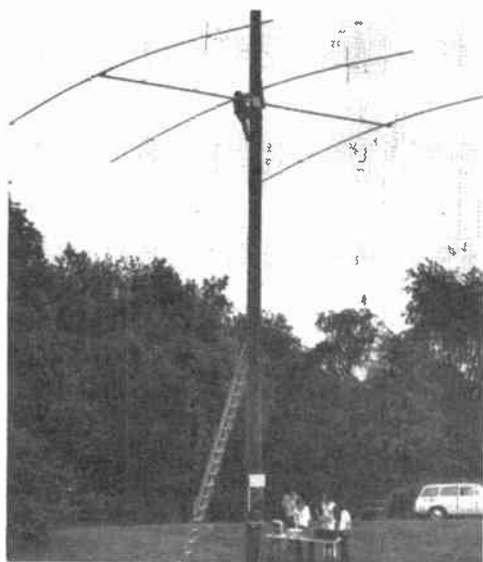
Fig. 1 — The short 40-meter Yagi resembles a large 20-meter system.
