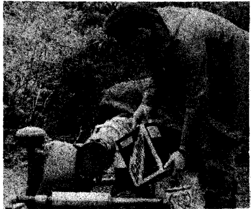
Fig. 10-5 — Gasoline-powered ac generators used for portable/emergency operation should be treated for ignition noise in the same manner as automobile engines are. The frame of the gas generator should be connected to an earth ground, and the entire unit should be situated as far from the operating position as possible. This will not only reduce ignition noise, but will minimize ambient noise from the power unit. (Shown here is K1GTK during Field Day operations.)
