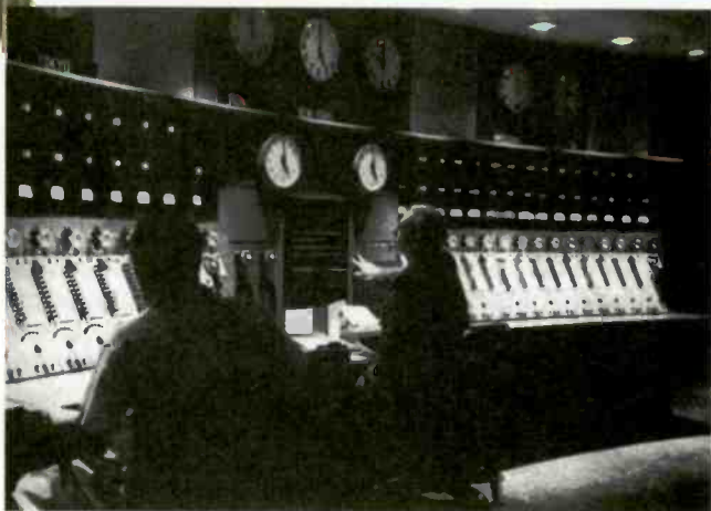
Twenty-six programs can be fed through the master control console simultaneously at Voice of America.
