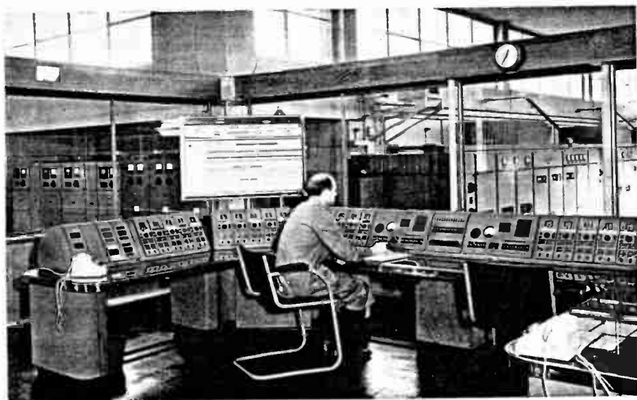
13. The central control positions at the G.P.O. radio station at Rugby
