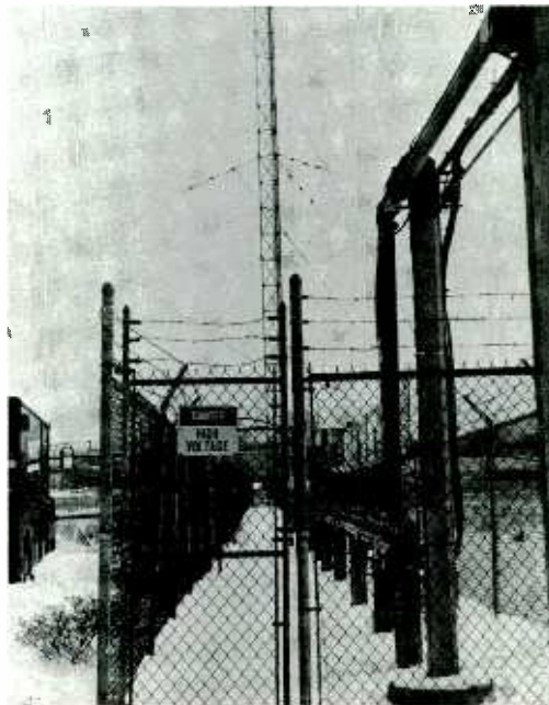
FIGURE 10.6 Lines leading from station transmitter to antenna base. FCC rules require fencing for safety purposes.
