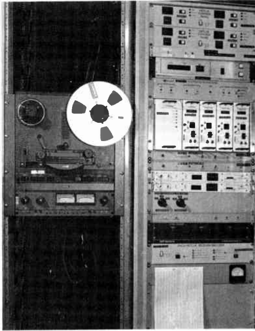
Figure 14.8 Equipment rack in a radio station.
