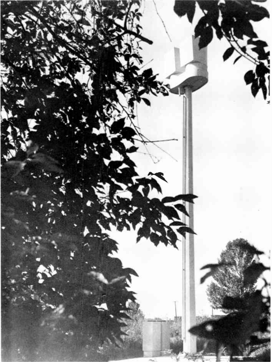
This is a more modern version of a microwave tower and antenna capable of transmitting many signals. (Bell Laboratories.)
