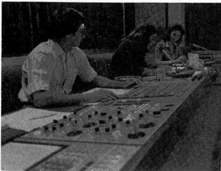
Fig. 1-3. View of a television control room.
