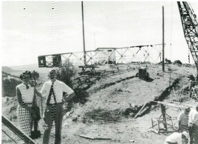
Sidewalk superintendents: The author and his daughter, Diane, watch a transmitting tower being erected on the peak of Mount Dufferin, west of Kamloops. It was a mystery to me that our engineering staff ever managed to get all the iron and steel material up the rugged mountain side, let alone erect it.
