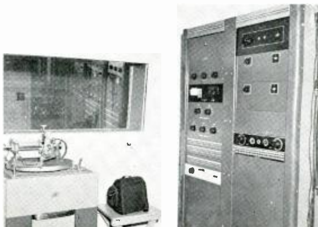
Patch panel and switch selector panels in recording room. Disc recorder is at left and small wire recorder at right under case.
