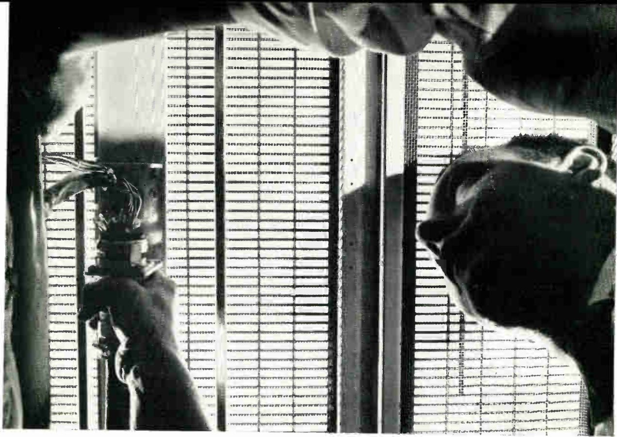
Customer engineer hooks up power cables inside the main frame while installing a computer system.
