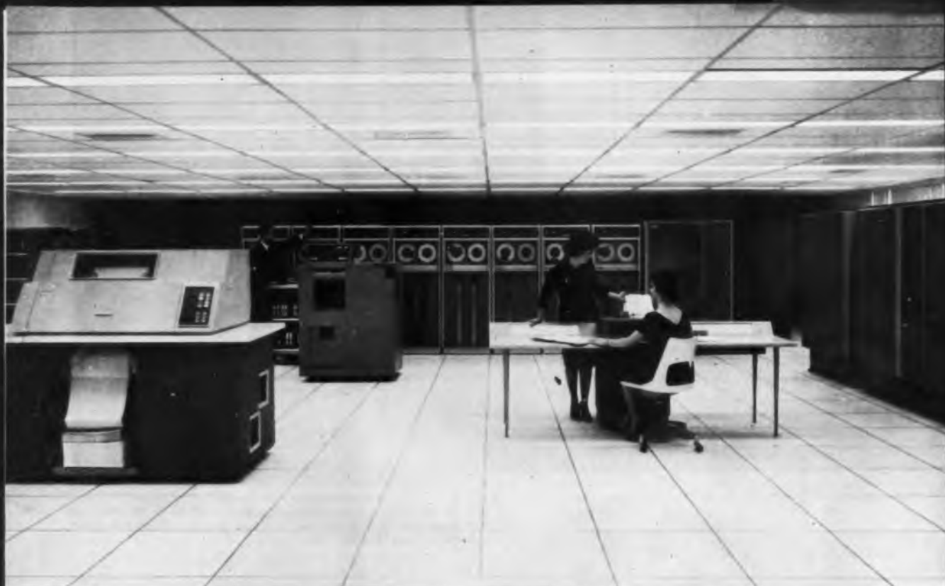
This Honeywell installation shows an output printing unit in the foreground (left). The reams of paper folding in continuous flow indicate the volume of data in process.
