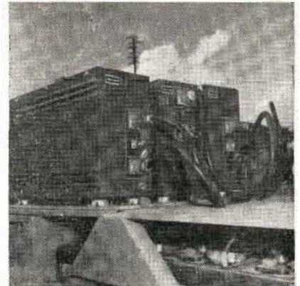
Fig. 2: Power equipment mounts above batteries
