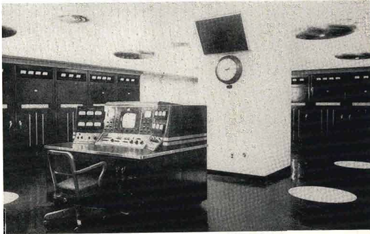
Fig. 1: WABD's operating console affords convenient view of the transmitter racks seen at the left
