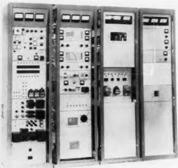
Fig. 4: The transmitter is housed in 4 cabinets; plate transformers for power amplifier are in an external, wire-screened enclosed area.
