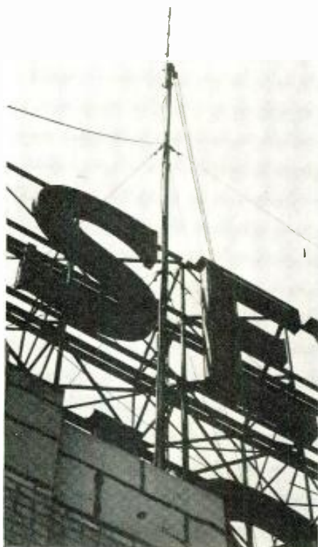
Fig. 3: Triple skirted, vertically polarized, coaxial antenna for mobile radio transmission atop the Essex House in New York City
