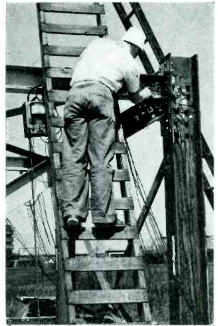
Testing strain gages during preparation for stress measurements on 80 ft. welded trusses
