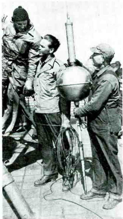
The flagpole ornament has nothing to do with the coax antenna being installed for West Coast cross-bay radiophone system
