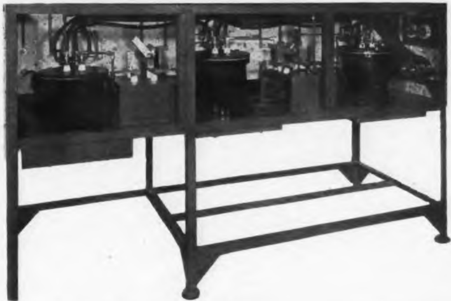
Fig. 4. Back view of switching unit which enables oscillator to be used continuously among three work-coil setups. Switching is in primary side of output transformers
