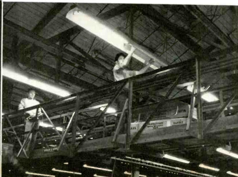
Servicing 18,000 fluorescents in Vega Aircraft, Burbank, Calif., plant, is facilitated by lamping bridge towed by monorail crane
