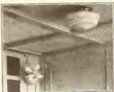
Efficiently equipped Demonstrating Room, showing Unico Lighting and Ventilating Units Installed. Comfort to your customer brings greater record sales.
