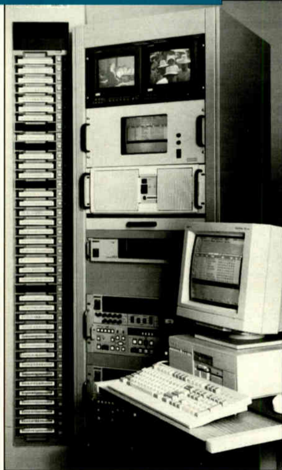
CFCN uses the Louth ADC-100 at its Calgary and Lethbridge stations.
