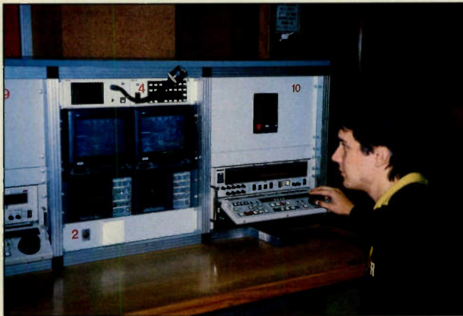
An operator monitors equipment in a control room at Televizija Slovenija.
