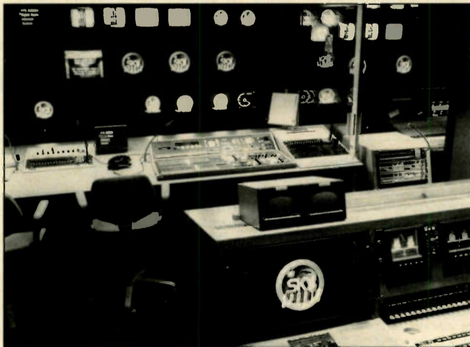
British Sky Broadcasting's Studio 5 Control Room boasts four RTS/Telex KP97 keypanels.
