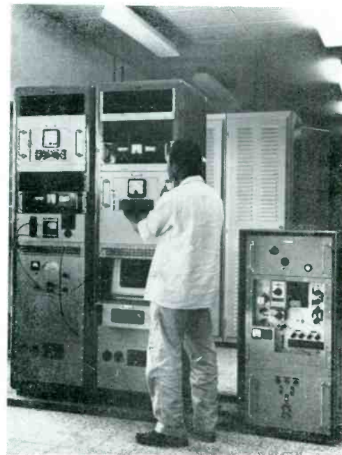
The Western Nigerian Broadcasting Service has been equipped with Redifon transmitters, and the illustration shows the VHF programme link equipment at Abafon. The racks contain, not only FM receivers, but amplifiers and test equipment
