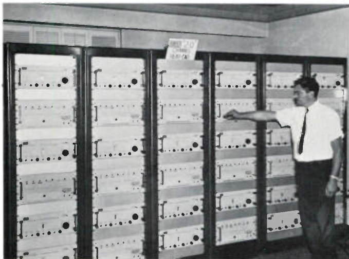
This 20-channel head-end installation was hurriedly installed by Jerrold and used to demonstrate that 20 programs can be telecast simultaneously.
