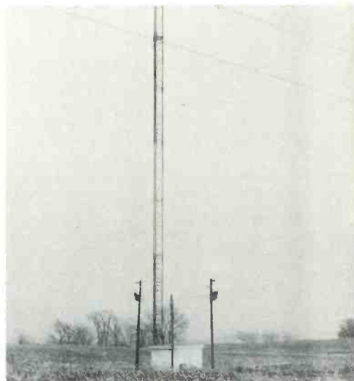
BASE of the Olivia 450 foot tower and the translator shack in a snow and windswept field in western Minnesota. Shack houses three UHF translators, associated amplifiers and test equipment.
