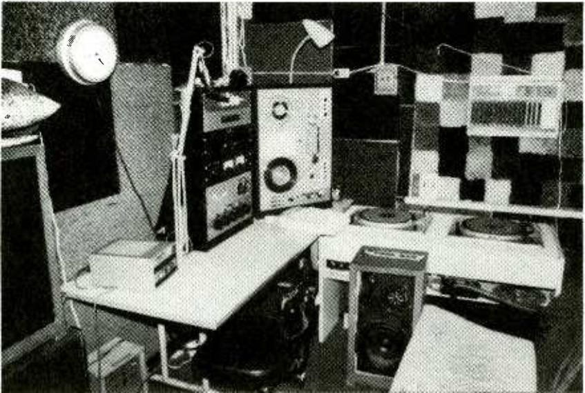
Emergency Control Room near transmitters
