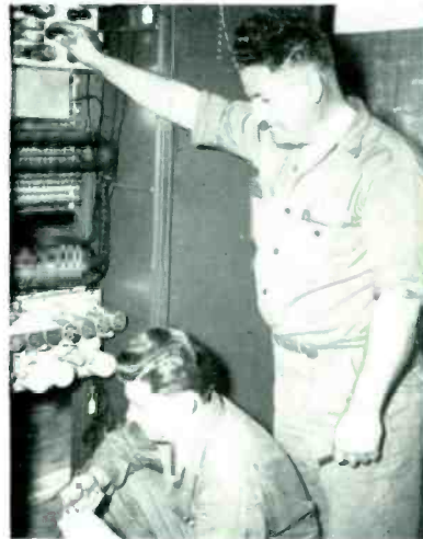
James Dennis and Garland Garthright were captured by the camera during the installation of WRVC's FM transmitter. Dennis handles remote pickups for WRVA in Tidewater.
