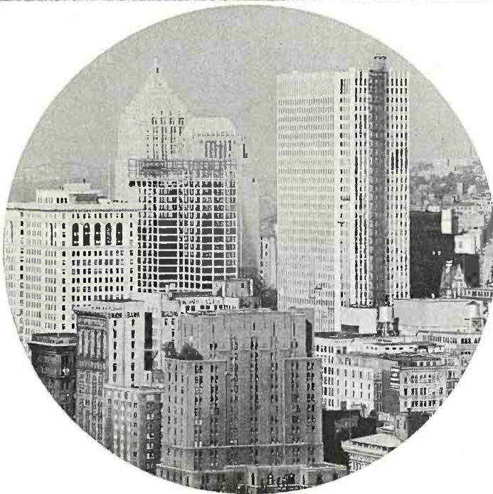
Our rapidly changing skyline looked like this when the Alco building was under construction.
