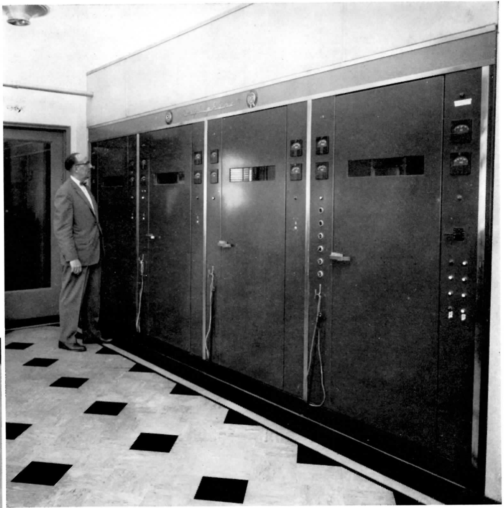
FIG. 24. WGN uses BTA-50G 50 kw Ampliphase transmitter. (It occupies same area required by former 10 kw transmitter.) Radio transmitter is remotely controlled 24 hours a day. (Shown is G. William Lang, Chief Engineer, WGN Radio.)
