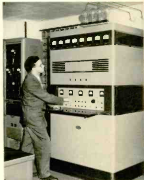
Engineer Charles Halle makes an adjustment in the transmitter controls. A technician with the signal corps during the war, Charlie is an experienced engineer. Like most radiomen, he operates his own amateur station.
