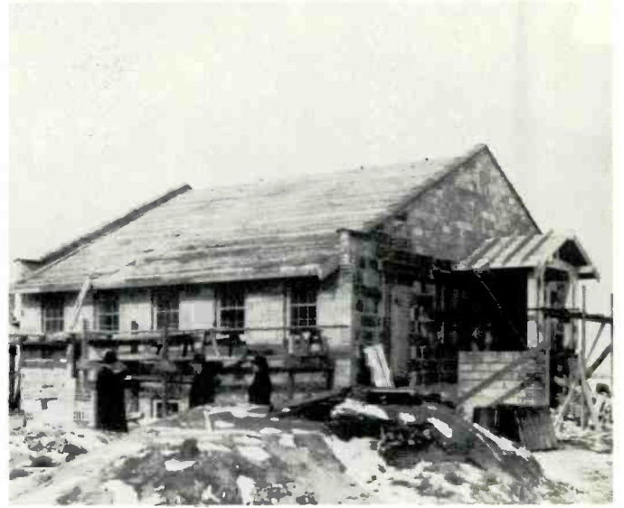
Following the ground-breaking, construction proceeded swiftly on the new WCCO transmitter building at Anoka. This mid-winter scene shows the progress that had been made early in 1925.
