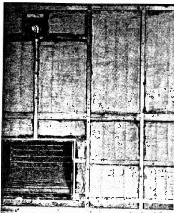
Figure 11. Application of acoustical treatment, showing rockwool blanket between wooden uprights. Observe the sound absorbing lining in the duct at the left.
