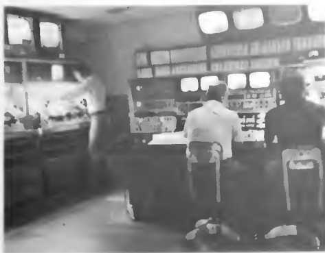
The control room is the pulse center of KMED-TV, handling the dissemination of network programs, locally originated programs, as well as the production of many local commercials.
